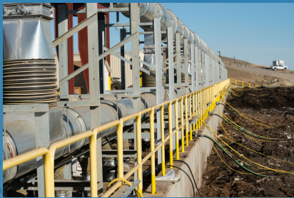
Yolo County Compost Landfilling is a stationary source within the District which received a PTO in 2022.
