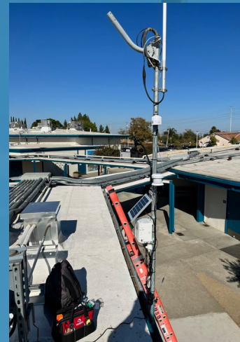
New weather and air monitor installed at Markham Elementary in Vacaville.
